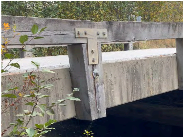
Cracked and rotten post rails
